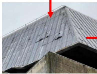
Vertical lead clad mansard surrounding the roof area, visible from street level
